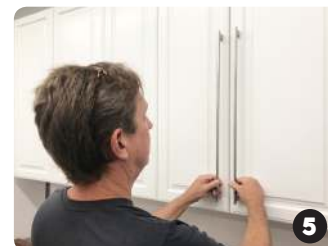
Position hardware by hand to find where you like it and mark position of bottom hole
